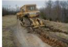
Figure 2. A dozer is ripping to loosen soils and produce soil conditions favorable to successful reforestation in a former roadway.
